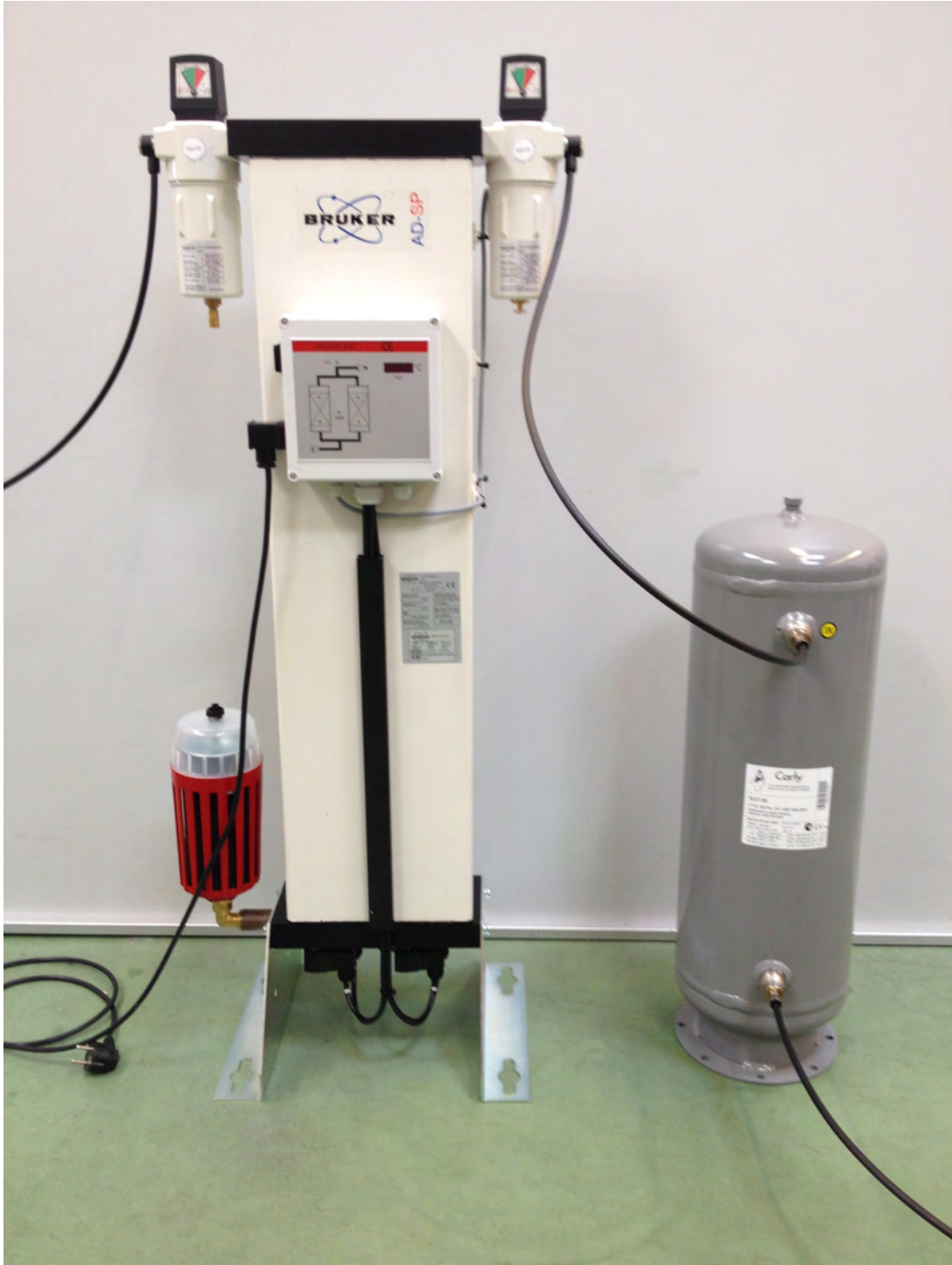
Figure 3.1: AD-SP Drier Installed with Buffer Tank
