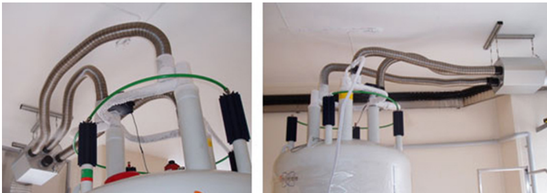
Figure 8.2: Emergency Quench Pipes
