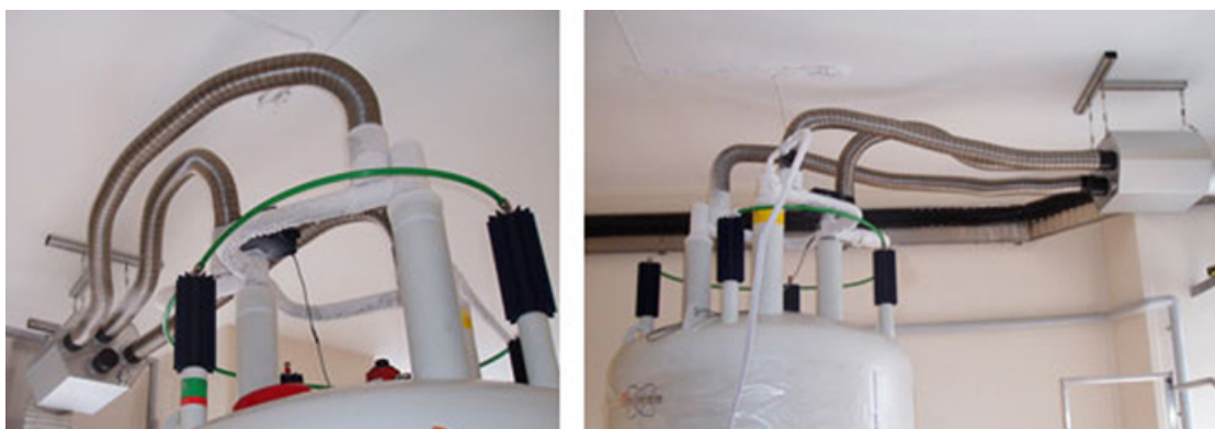
Figure 8.2: Emergency Quench Pipes
