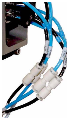
Figure 3.24. The labels of the hoses
